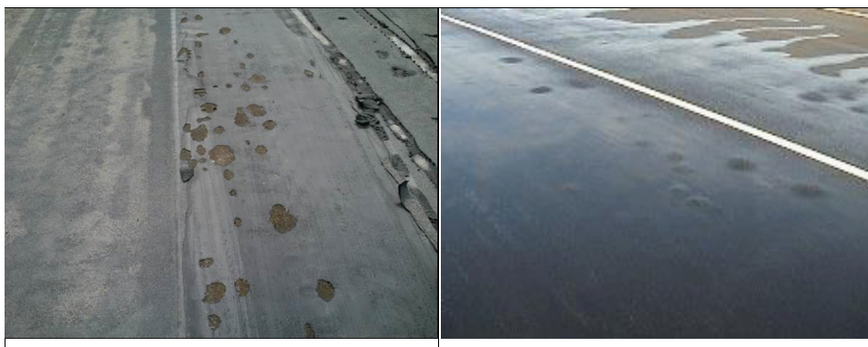
Fig. 1 Blisters containing gas on a) the waterproofing membrane b) the asphalt pavement
