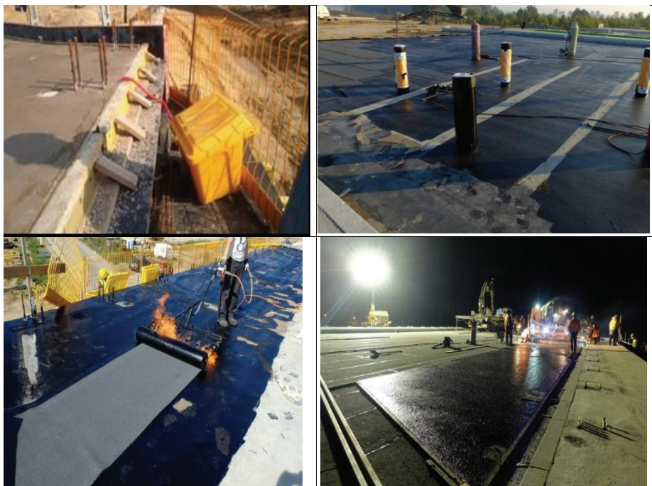
Fig.4 The pavement construction. Sensors fixed inside the deck and put into the box, which contained the data acquisition devices. Visible location of the sensors on the surface; they'rey stripes on a primer black background.
