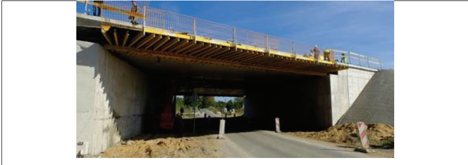
Fig.2 The view of the bridge deck at the A2 carriageway under construction.
